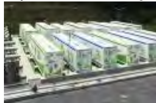
Battery Storage Installations
