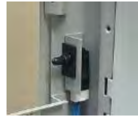
Door Switch in Access Level 2
