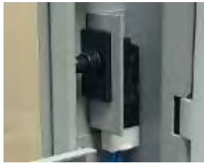
Door Switch in Access Level 1
