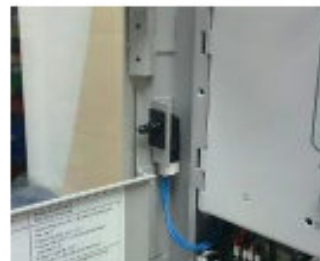
Door Switch in Access Level 2
