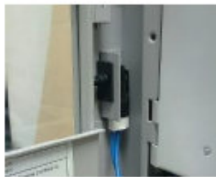
Door Switch in Access Level 1
